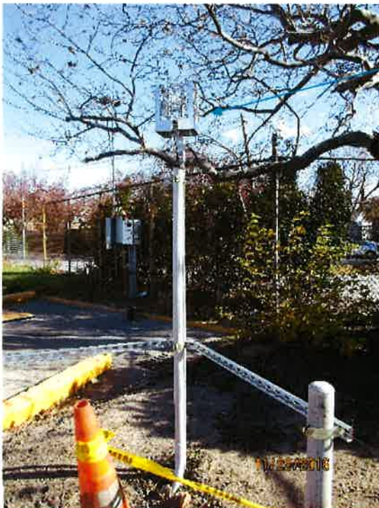
Photograph 2 – Solar powered wet sensor electronic housing
