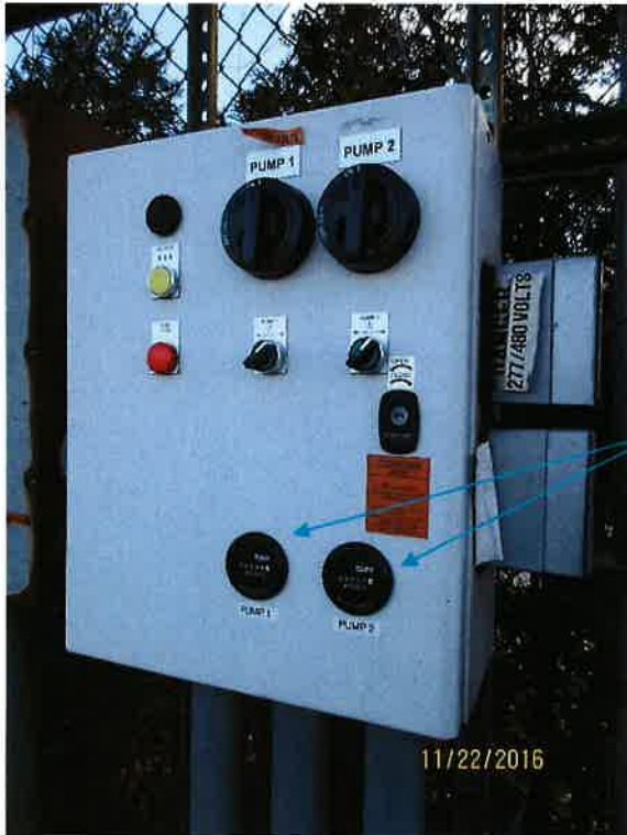
Photograph 1 – Pump run-time meters
